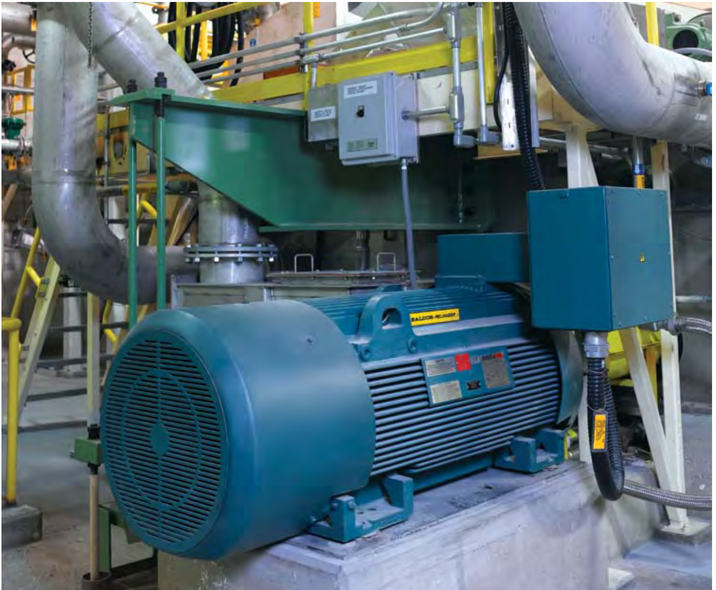
This Baldor•Reliance 200 HP AC motor was engineered for SCA for this specific screening application. The motor base speed is 720 RPM and is driven by a variable frequency drive, helping SCA save energy.
